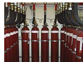
Gas Suppression Systems
